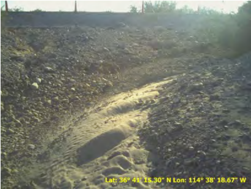
Photo 10. M06 Channel scour caused by runoff from SH 168 (background).
