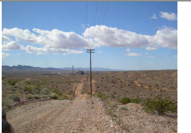
View south of the transmission line located on the western portion of the Subject Property.
